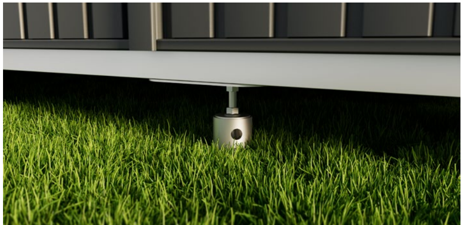
Fixing the Berry aluminium bottom frame profile to uneven ground with screw foundation
