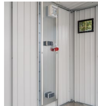
Electrical panel incl. sockets, LED lighting and optional high-voltage connection Width x height: 47 x 180 cm
